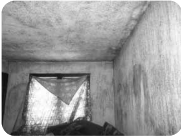
Atypical condensation; get a contractor!
